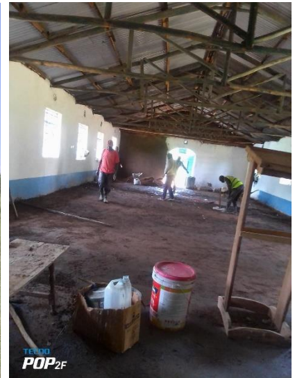
Floor Laid Last Week and Building Painted—Will Be Housing for 150 Boys at Next Youth Conference
